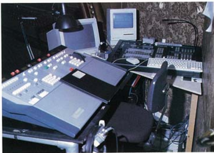
A view of the control desk which for the first time in Haymarket history has actually made it to a front of house position in the corner of the balcony. The Macintosh runs 'Light Talk' for the six Digital Light Curtains, whilst the Mini-Artisan controls the 18 VL5s.
